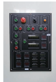
< Control System Equipment >
